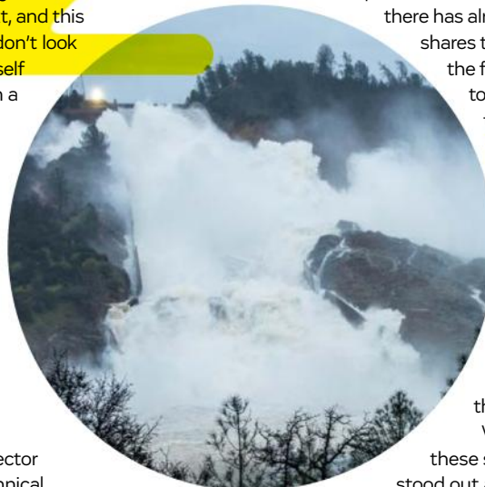
Water moving down the damaged spillway at the Oroville Dam on 17 February in Oroville, California.
